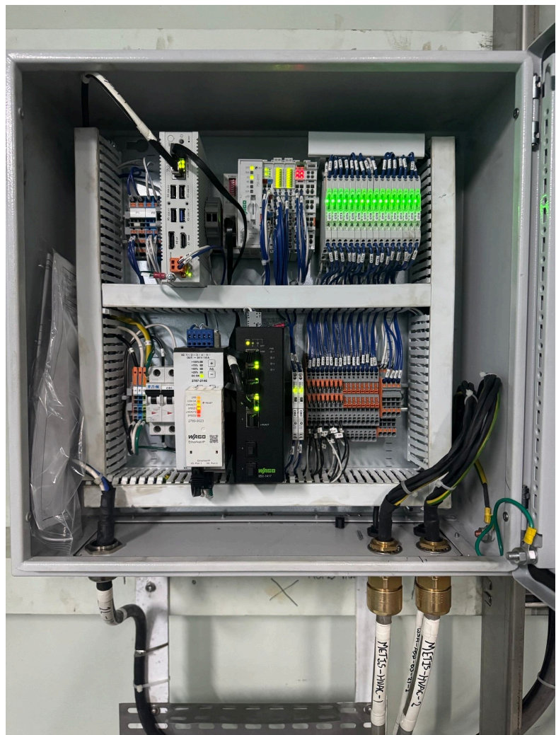
The WAGO edge compute enclosure installed aboard West Saturn, running the containerized Metis stack.
